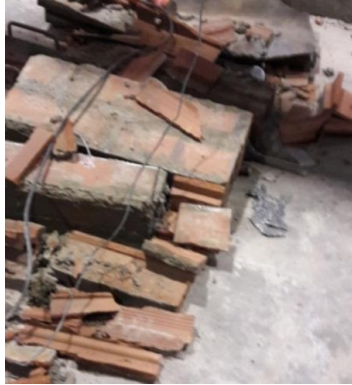
Plate 4.2: Failure patterns of Clay bricks wall
