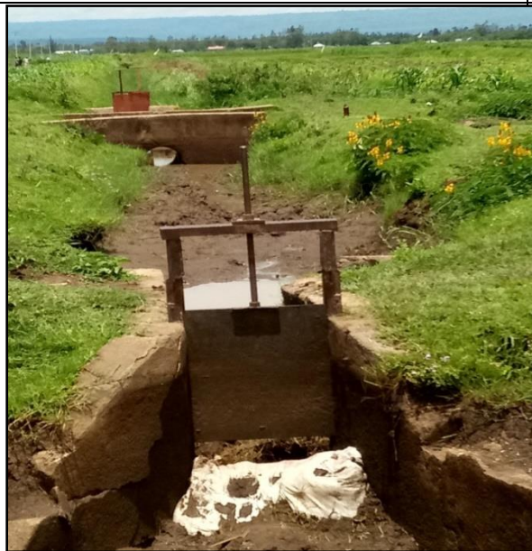
(c) Broken gate in Ahero irrigation scheme
